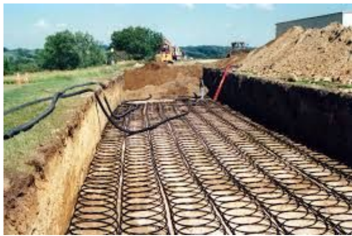
Geothermal Heat Pump
